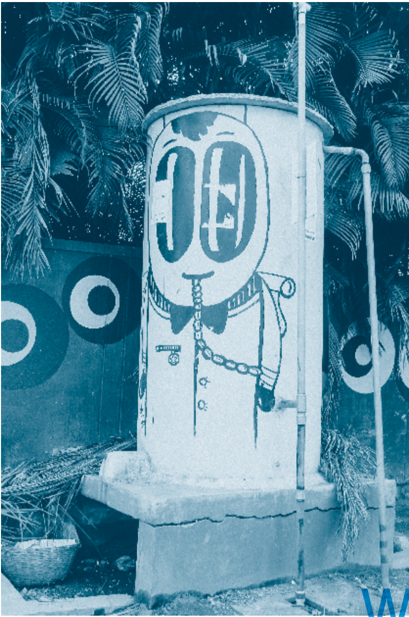
A water tank connected to a borewell
