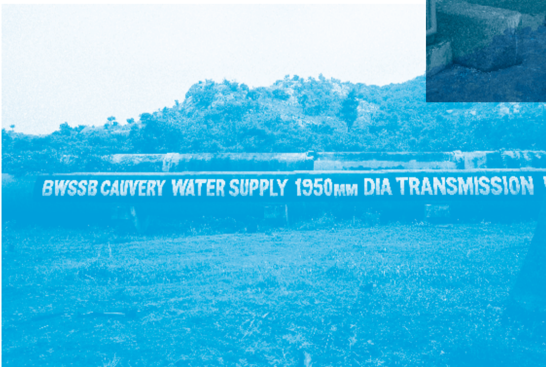
Cauvery Supply lines to Bangalore
